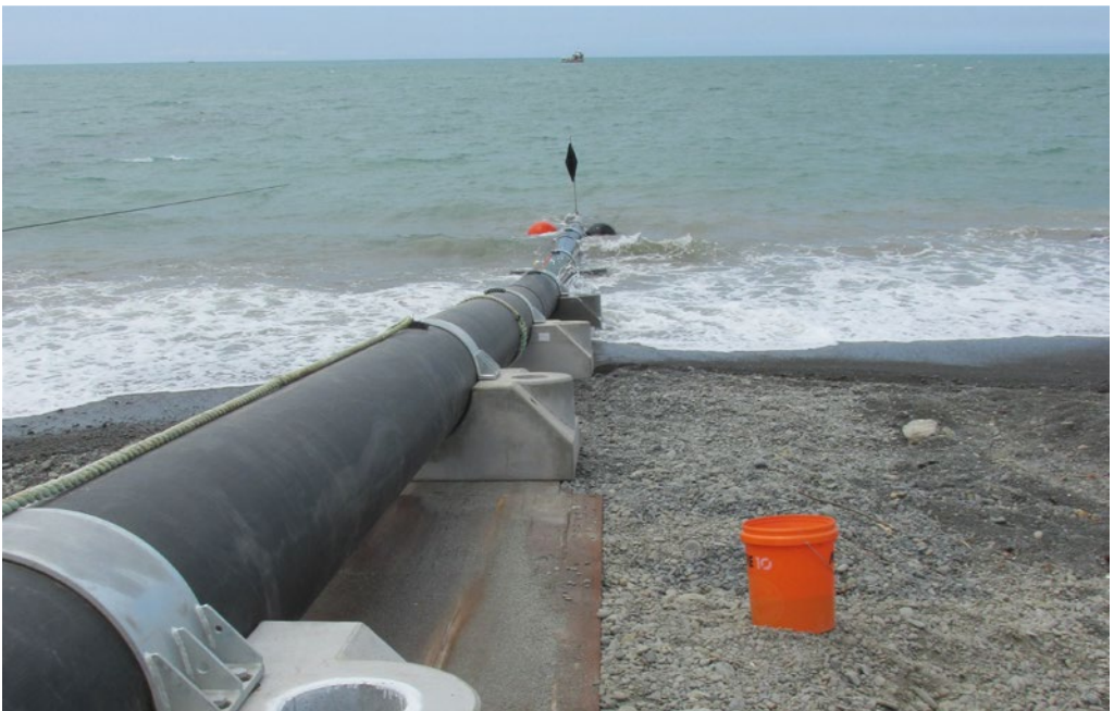
Top & Above: The first 200-metre length of the treated wastewater pipeline extension being deployed in December 2017.
