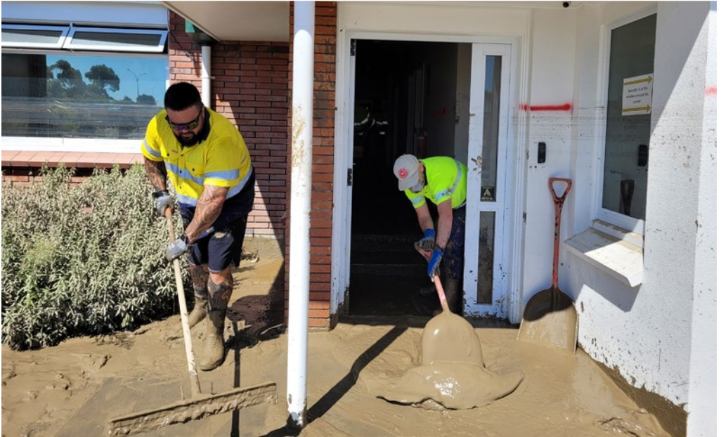
Top : The effects of Cyclone Gabrielle on the Whirinaki site, February 2023. Above: Cleaning silt out of the Security building.
